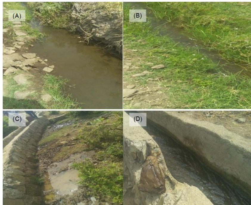
Figure 2. Consequences of water loss in the main canal (A), growth of grasses and weeds (B), seepage loss (C), and unauthorized water turnout by farmers (D), during the field campaign in December 2023.
